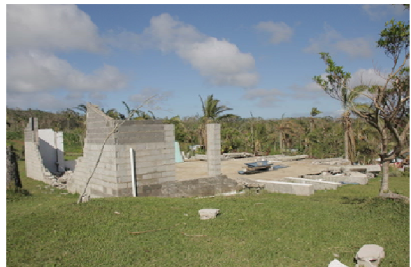
Figure 5. Collapsed church building in Green Hill.
